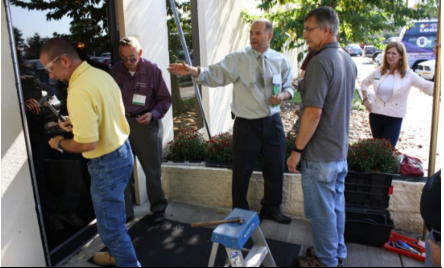
GPLA President Cliff Shafer instructs the installation of the R2 VARYX continuous hinge at the Philadelphia Hilton Hotel. R2 Hinge CEO Kerry Sprick (far right) observes the install.
